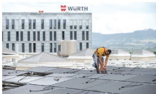
Adolf Würth GmbH & Co. KG plans to build photovoltaic systems on a total surface area of up to 28,000 m 2 in the final construction stage on the campus in Künzelsau and the nearby logistics hub in Gewerbepark Hohenlohe industrial park in 2022.
